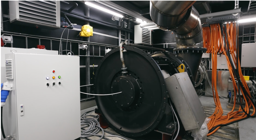
Figure 6 One MW turbo blower under tests
