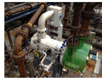
Figure 14 – ICML during Factory Testing
