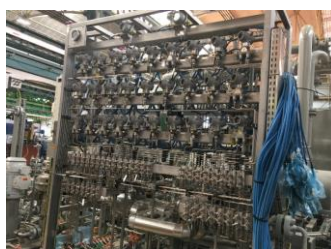
Figure 10 - DGS Monitoring Panel
