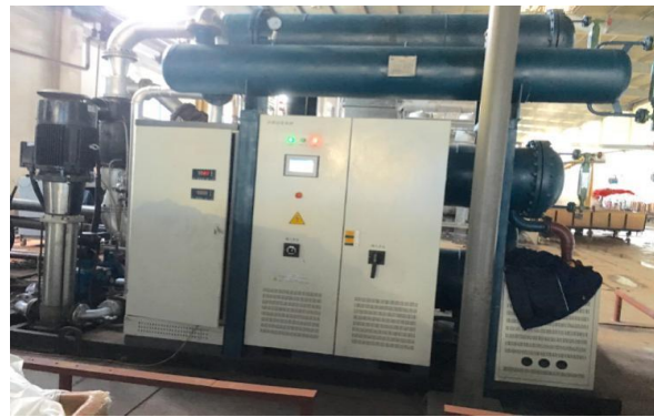
Figure 16. Application of ORC waste heat generator supported by permanent magnetic gas suspension bearing
