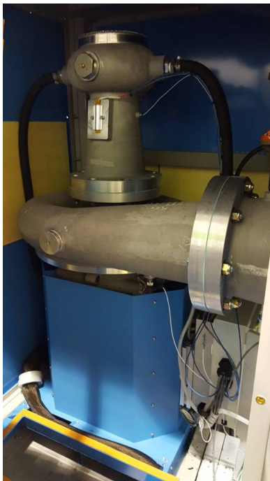
Fig. 15: Core machine installed in cabinet with inlet venturi and cooling shroud.
