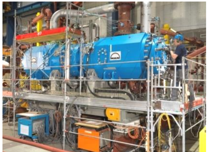
Fig. 5: Installation of HOFIM compressor in the test bed (picture by MAN).
