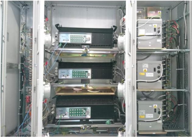
Fig. 5 AMB control cabinet during commissioning.
