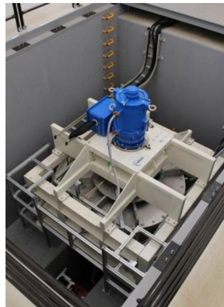
(b) The FESS demonstration machine installed in underground storage space
