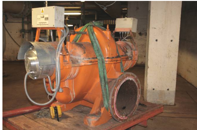
These components were maintained, repaired respectively renewed due to their condition. Fig. 2: AMB supported coolant pump after long term operation
