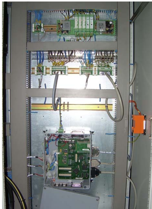
Fig. 11: Control electronics mounted in an electric cabinet
