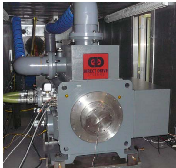
Figure 1. 1MW 15kRPM PM Motor on Magnetic Bearings.
