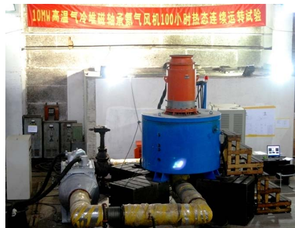
FIGURE 3: Picture of the test loop for the HTR-10 helium circulator
