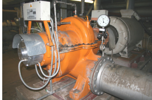
FIGURE 3: AMB-pump operating in the power plant
