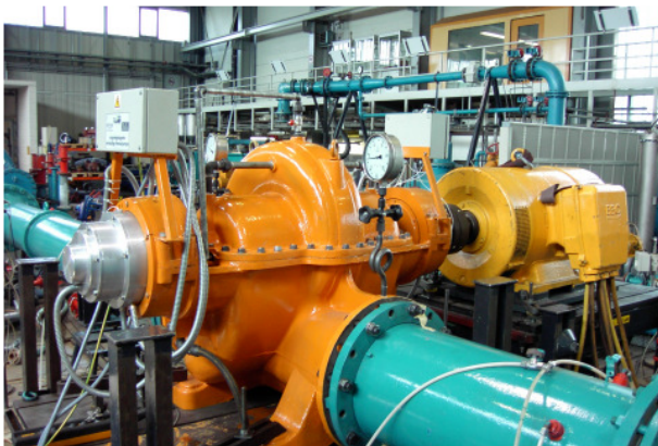
FIGURE 2: Pump in the flow-loop-test-bed at KSB
