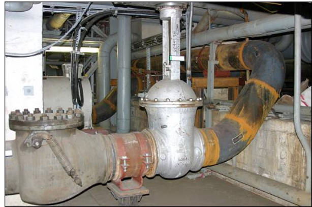
FIGURE 15: Non-return valve and slider in the pressure line
