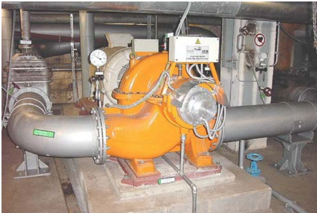
Fig. 5 Pump SM 400/400 installed in the Power Station
